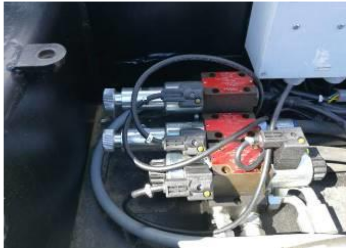
Picture 15. Valves under the cover
